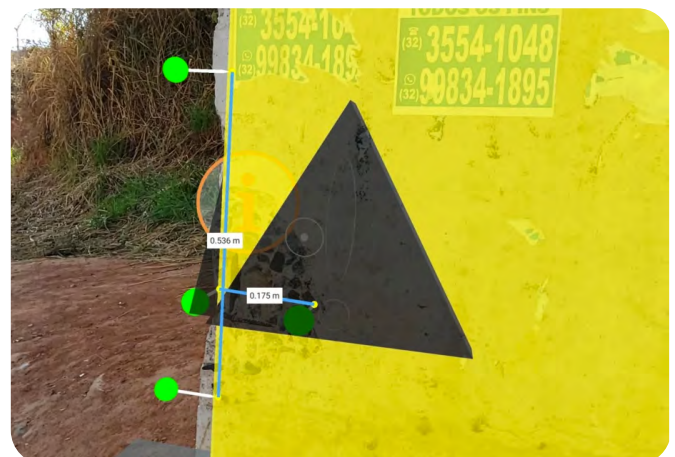
Documenting concrete spalling damage measurements on-site using GAMMA AR to inform maintenance and repair decisions.
