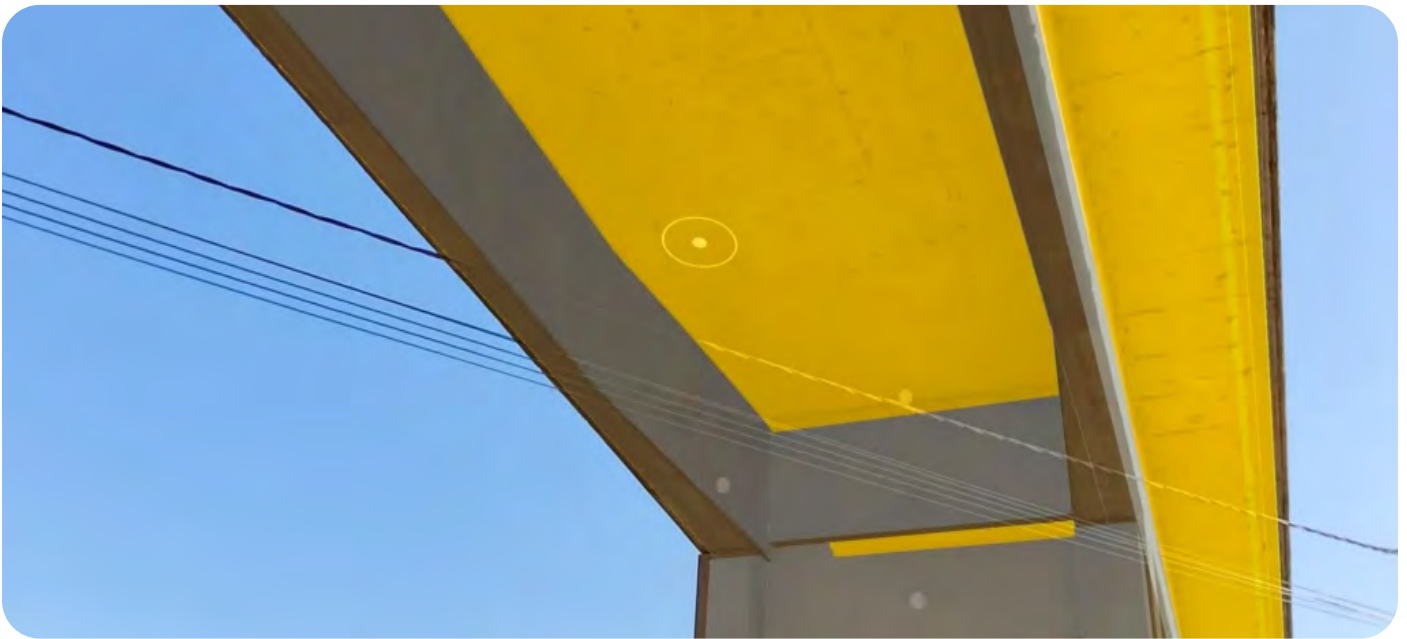
GAMMA AR overlay of the BIM model onto the physical bridge for identification and documentation of damage.
